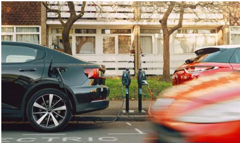
An example of an on-street residential parking charger (picture from West Sussex County Council)
